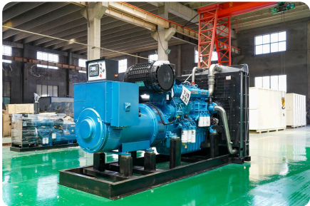
Sets in the test bay.
